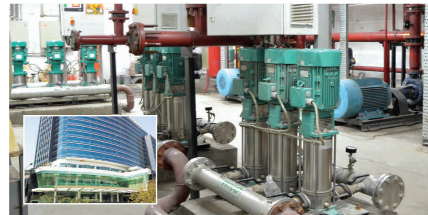
Supply: 6 Nos pressure boosting systems 22 Nos dewatering/ sewage submersible pumps 11 Nos control panels for dewatering/ sewage submersible pumps Client: Hotel Sofitel, Mumbai
