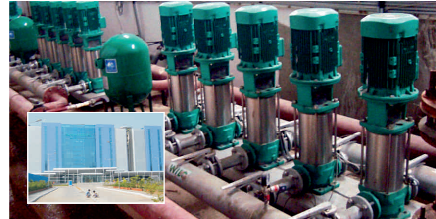
Supply: 7 Nos pressure boosting system 12 Nos dewatering/ sewage submersible pumps 6 Nos control panels for dewatering/ sewage submersible pumps 24 Nos HVAC pumpsets 4 Nos Fire fighting pumps sets Client: Seven Hills Hospital, Mumbai
